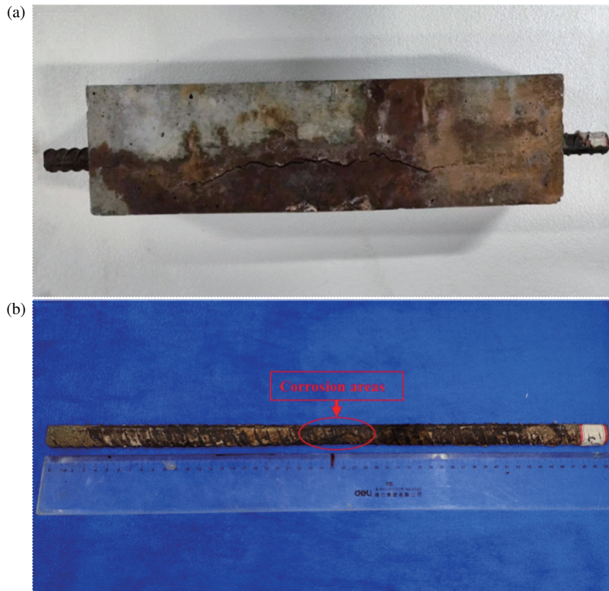
FIGURE 8. Actual results: (a) Corroded reinforced concrete; (b) Corroded rebar within concrete.
