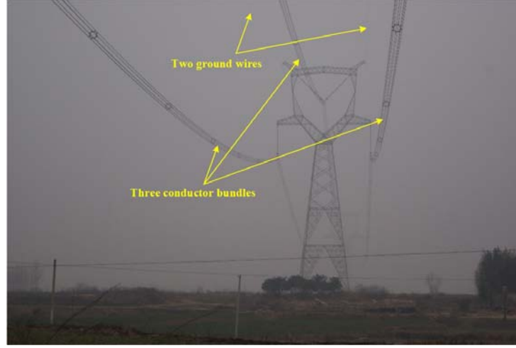
Figure 2. Photograph of Jindongnan-Nanyang-Jingmen UHV transmission line in Hubei Province. Three conductor bundles and two ground wires are hung on the cat-head-shaped pylon.
