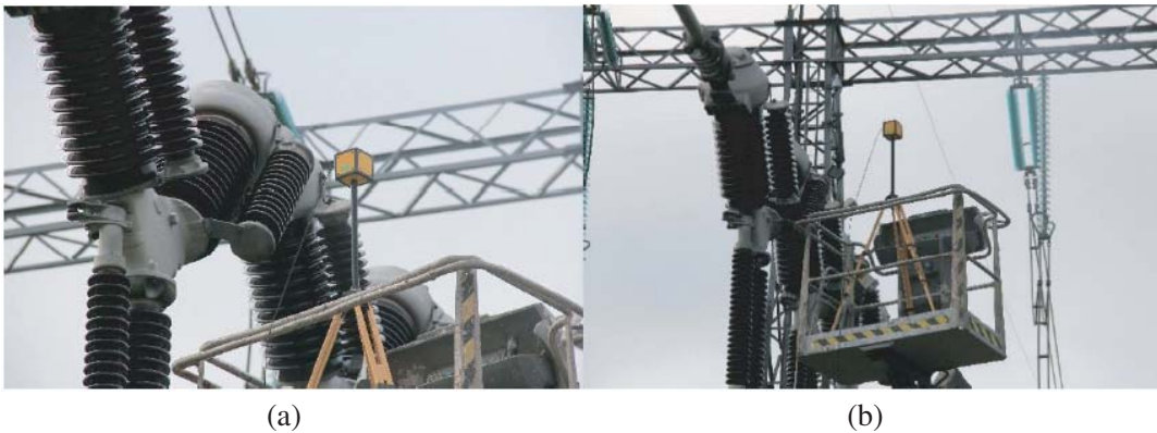
Figure 4. Measurements close to a breaker pole with the probe at (a) 6.83 m and (b) 7.63 m (horizontal distance from pole to man hoist center approx. 1 m). Note: The presence of capacitors and the fact that man hoist movements could not be controlled with extreme precision placed limitations on how close the man hoist could be moved to the circuit breaker.
