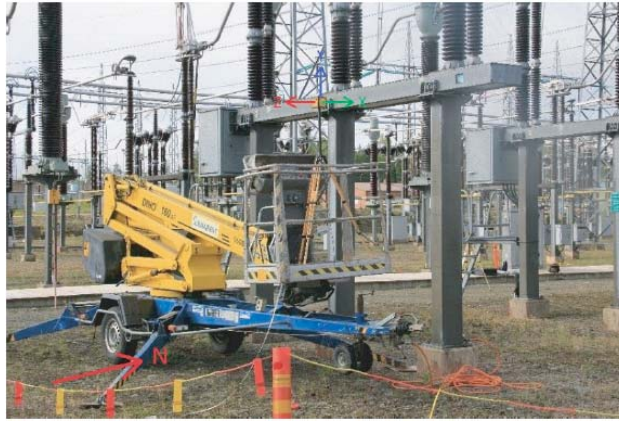
Figure 5. Man hoist “outside” the circuit breaker in the position where it can be moved to another location (man hoist/probe height 1.13/2.83 m).
