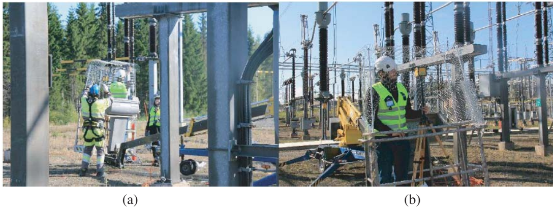
Figure 7. (a) The Faraday cage constructed on site to protect the man hoist, with the top net already in place and the cover being installed. (b) The cage and an opening down in the front.
