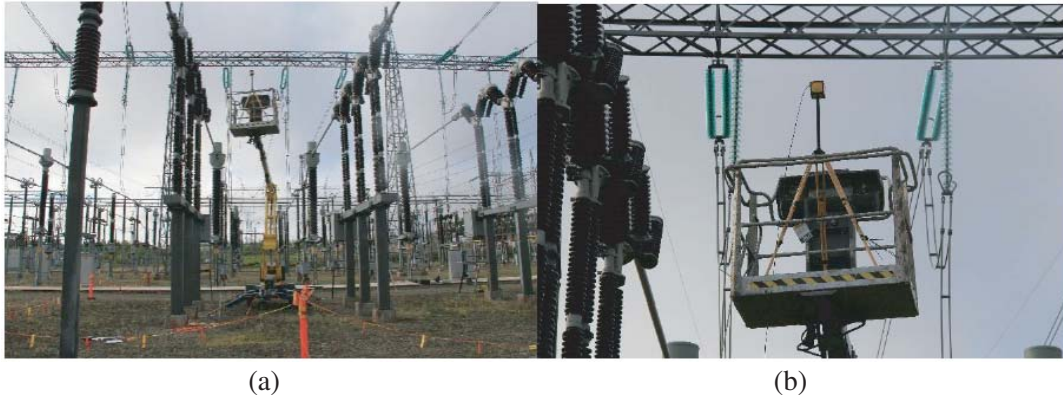
Figure 3. (a) Measurement between two phases with the probe at 6.83 m from the ground. (b) A closer view of the probe and the man hoist.
